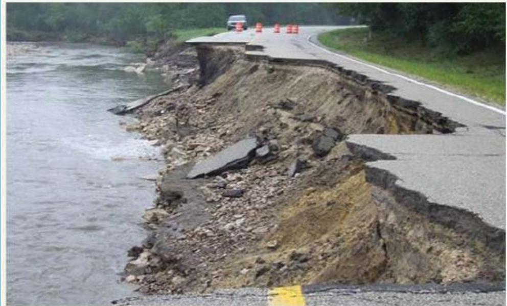
Fig. 1-11. Flood damage along Whitewater River exceeded $4 million at Whitewater State Park.
